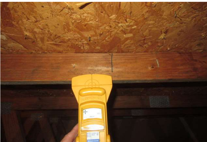
Nail location verified
